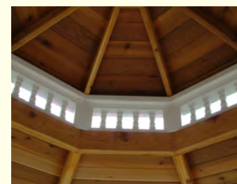
Picture of installed Spindles
